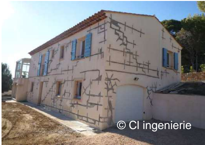
Fissuration des structures
